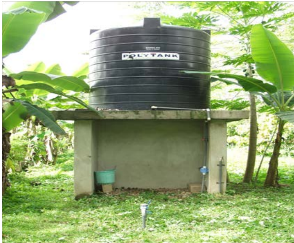
Plate 17 Water tank mounted on a raised concrete platform
